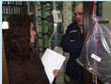
Area Manager, Pat Kearney discusses the logistics of the site connections to Project Administrator, Gail Hoyles while in New World Island.
